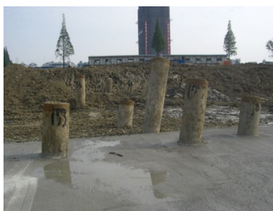
图 8 基坑开挖等施工原因造成管桩倾斜(沈国勤等 [9] ) Fig.8 Pipe pile inclination caused by excavation or construction(Shen Guo-qing [9] )
